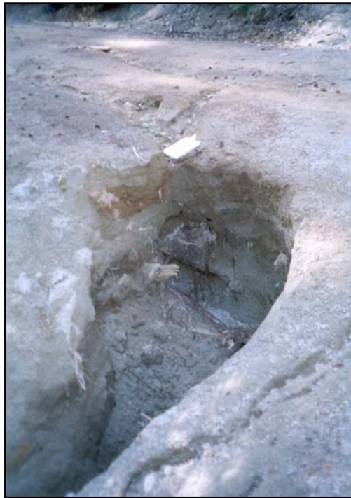
Figure 6. This bank erosion occurred on 22N25 during a normal precipitation year when concentrated surface drainage left the road at an inopportune location. The slump material was delivered to the RCA of Pinchard Creek, which is located less than 150 feet from the road. This road was reconstructed in 2003. (clipboard is shown for scale).
