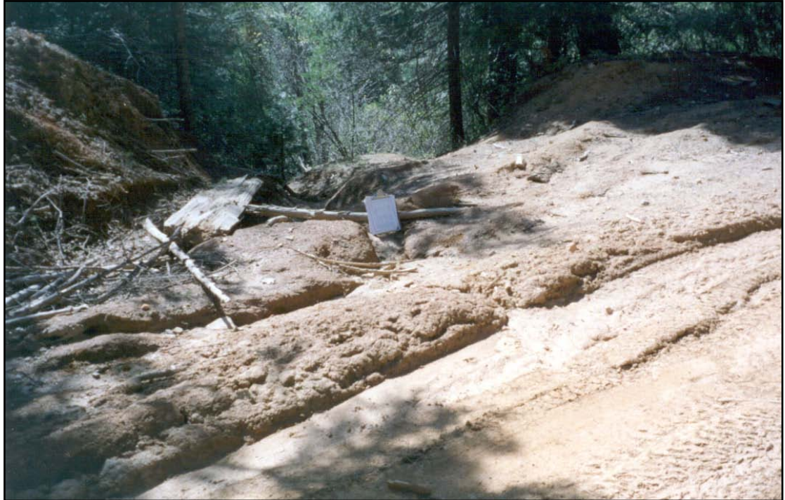
Figure 5. Due to infrequent cross drain spacing, the outlet of this rolling dip on 22N25 was badly eroding and delivered sediment off of the road to the neighboring riparian area. This road was reconstructed in 2003. (Clipboard is shown for scale).
