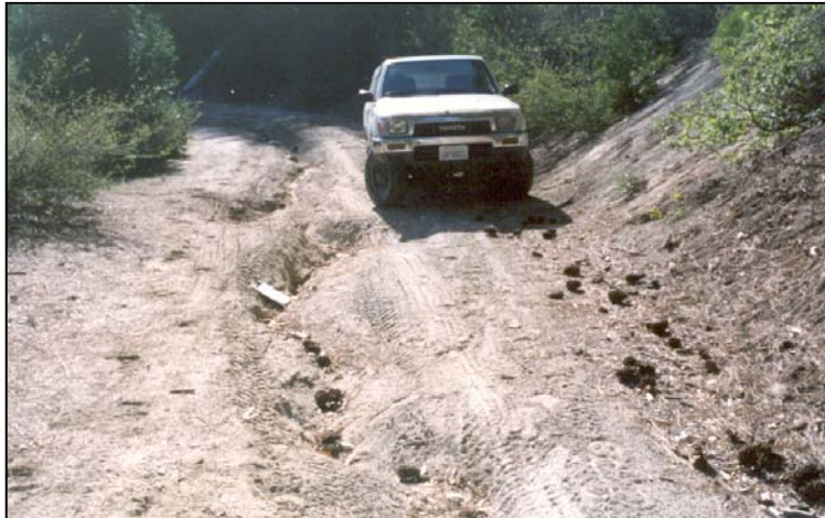
Figure 4. In 2002, Road 22N25 on Feather River Ranger District exhibits severe rutting as a result of a poorly drained surface that concentrates runoff. This road was reconstructed in 2003.
